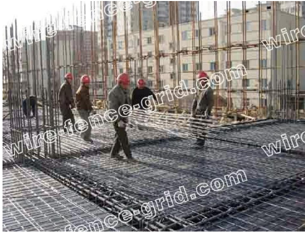
deformed weld mesh
