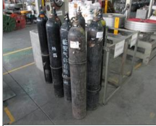
Photo of non-conformity Gas cylinders are not secured.JPG
