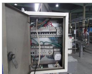
Photo of non-conformity Electrical panels in No. 2 production building were not installed with inner covers.JPG
