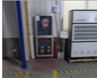
Photo of fire safety equipment Fire equipments.JPG
