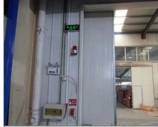
Photo of fire safety equipment Fire alarm.JPG
