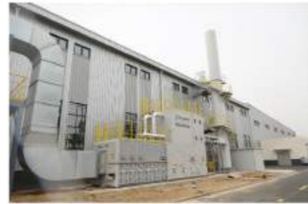
VOCs exhaust gas treatment
