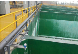
Liquid level inspection of tap water and sewage treatment
