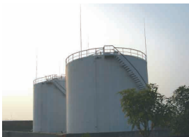
Oil-water interface measurement of oil depot system
