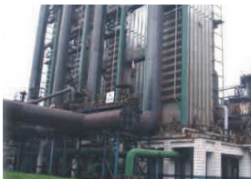
Tar-ammonia water interface measurement of coke industry
