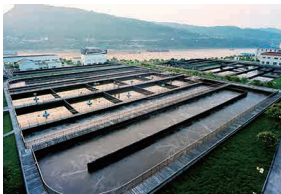
Urban water supply and sewage treatment
